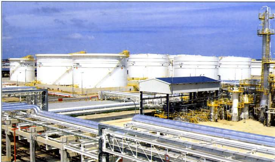
Storage tanks and pipelines at the Melaka refinery
